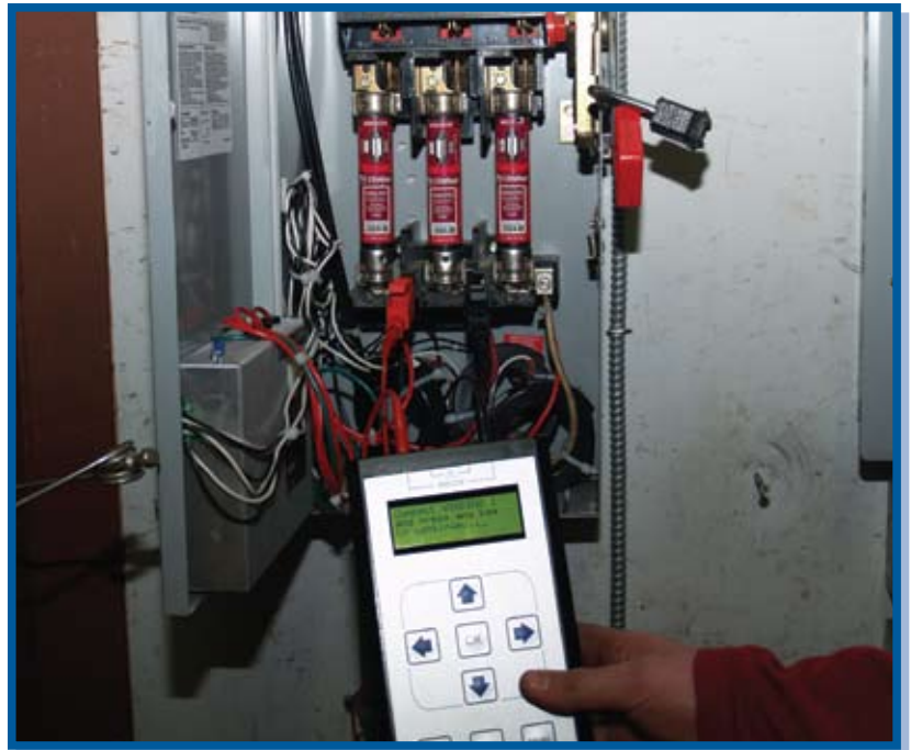
A 2-minute test from the MCC evaluates the windings, cabling, and connections through even hundreds of feet of cable.
